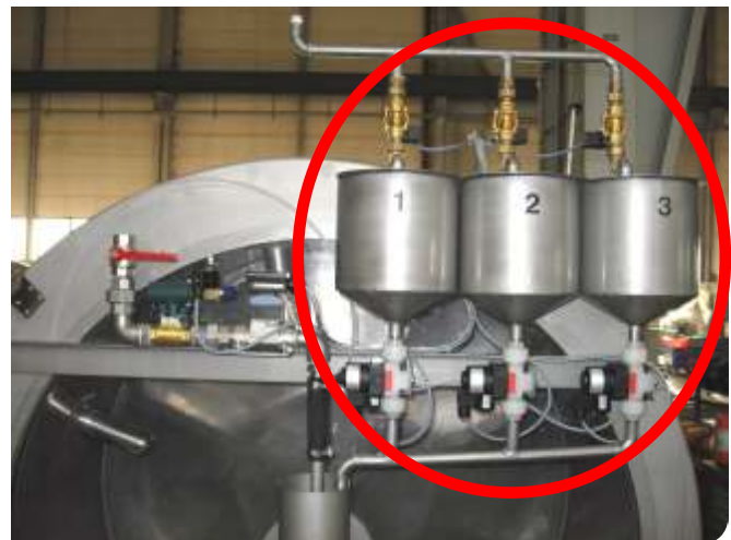
Chemical tank with automatic dosing
