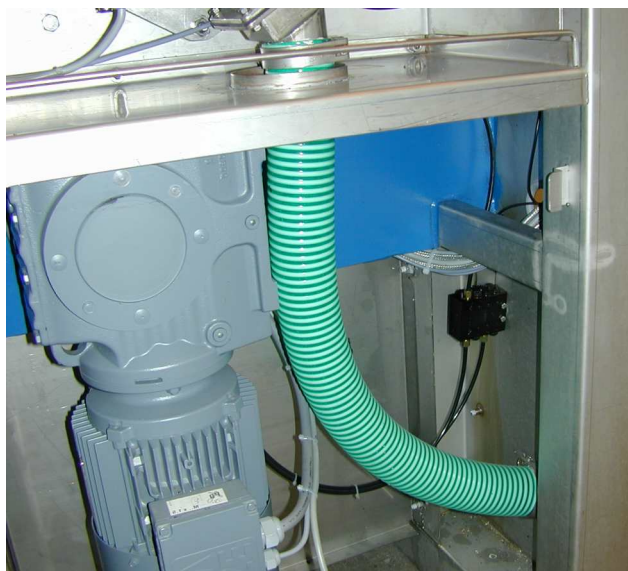
VG drive, draining pipe and central lubrication
